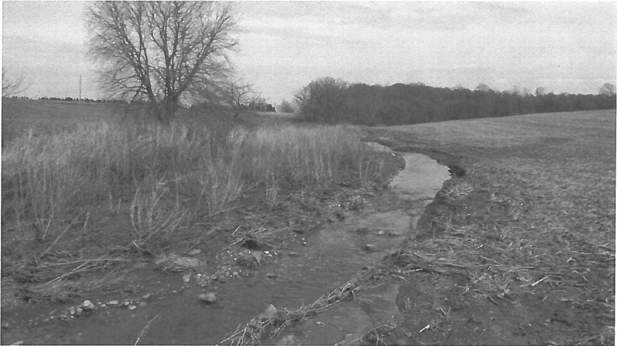
On center part of farm looking east (downstream) Existing ditch is on left in grass area - new ditch being created to south of existing ditch
