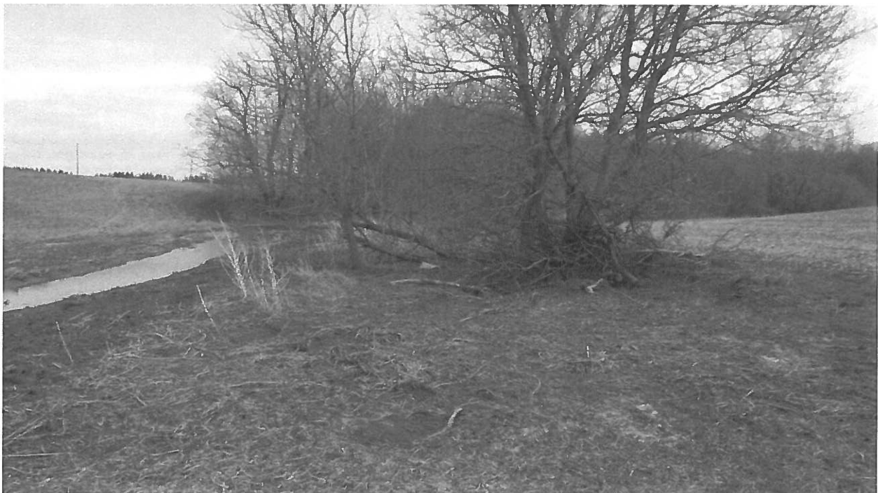
On east part of farm - standing in existing ditch area looking east (downstream) New ditch being created on north side of existing ditch
