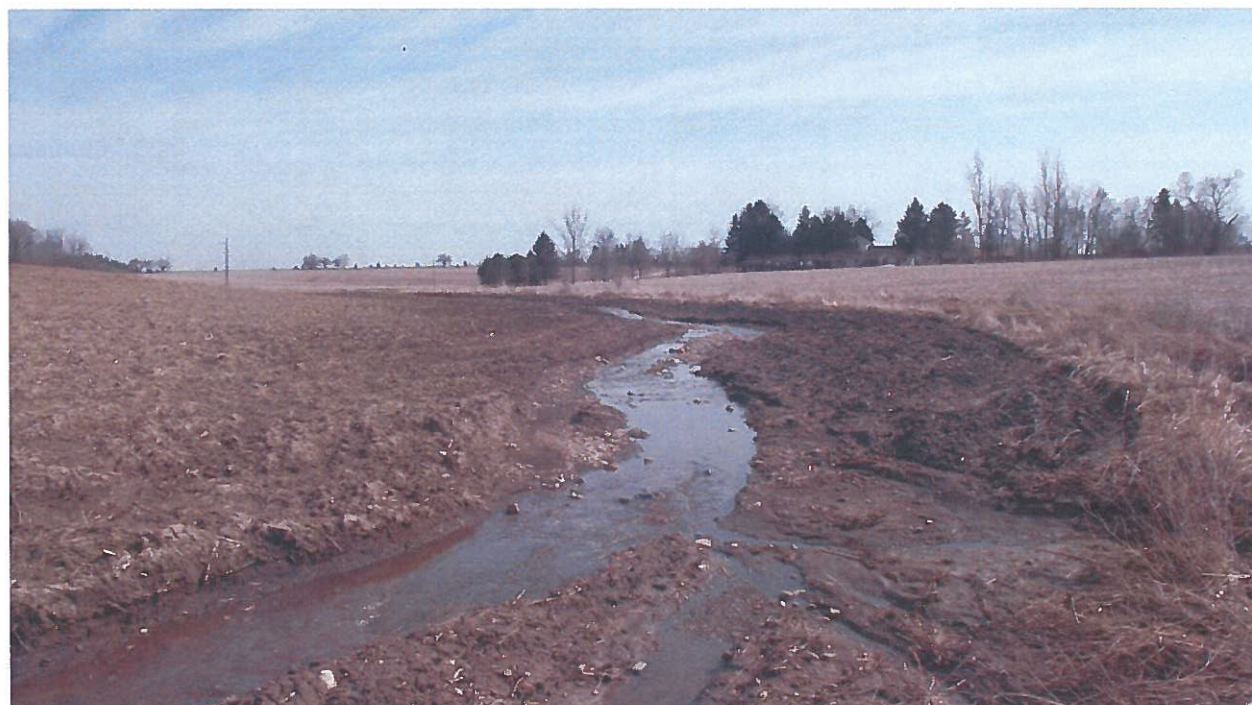
Looking downstream (northeast) toward Bean Road - existing ditch is to right New ditch being created on northwest side of existing ditch
